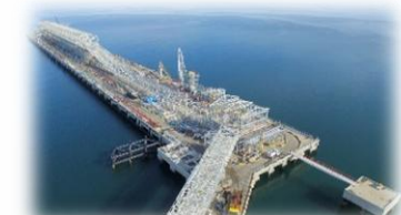
Samur Project At Sabah Malaysia, 1,120 TPH Portal Scrapper reclaimer, Conveying system and Ship loader
